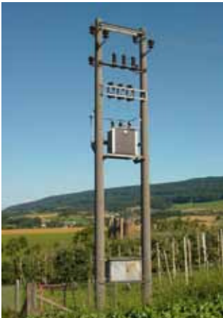
Stangenstation Stiigere, Freienwil
