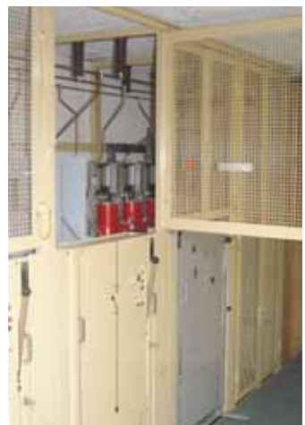
Transformatorstation Hofwies, Ehrendingen
